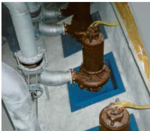
Sewage pumps installed dry.
